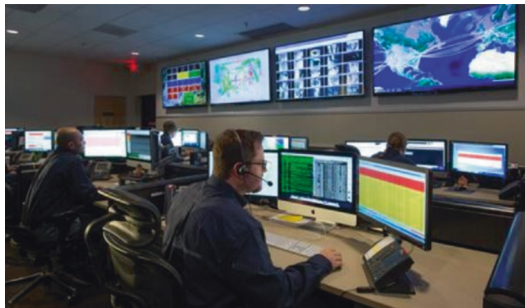
■ Fig. 15.3 Example of a Network Operations Center (NOC). (Image used by permission of NTT Ltd (available at ► https://www.gin.ntt.net/support-center/noc/ ))
